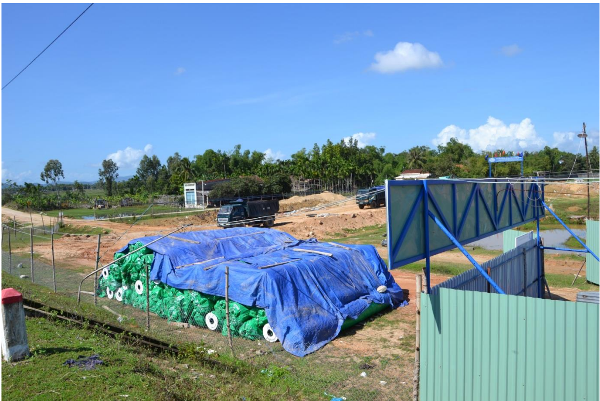
Figure 23 Construction of a wastewater plant in Tam Ky, financed by international donors in 2014/15
