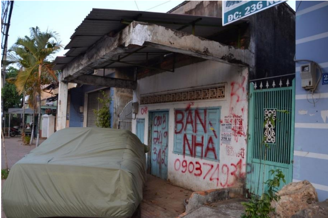
Figure 36 Abandoned house in Buôn Ma Thuột
